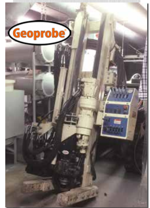
Set up inside a building with 9.5-ft. overhead clearance prior to drilling a 4-in. diameter SVE well using standard 5-ft. long, 6.25-in. ID HSA.
